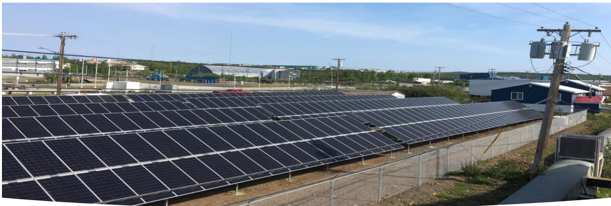
Pictured above: The completed Nihtat Energy Ltd. PV solar installation at Inuvik North Mart.
